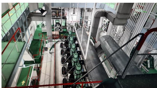
Figure 3. A view of the auxiliary engine in the marine engine room simulator.
